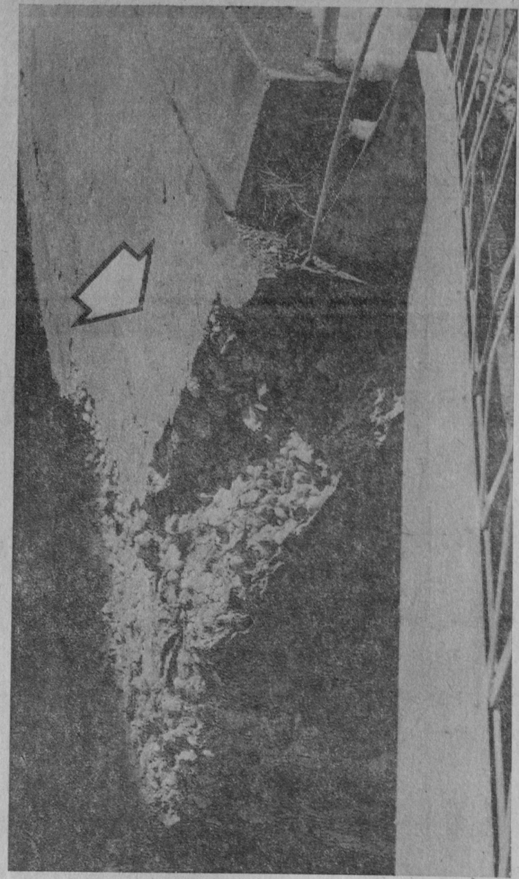
AN EXAMPLE of the deterioration of concrete abutments on Tawas City's bridges over the Tawas River is shown in this photograph. The arrow points to the facing edge of one abutment on the Whittemore Street bridge. Concrete is crumbling away from the area where steel girders rest on the abutment. Load limits have been lowered on this bridge to prohibit truck traffic.—Tawas Herald Photo.
