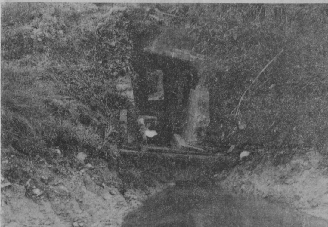
TRAFFIC at one point on the Detroit and Mackinac Railway has been slowed to a snail's pace—three miles per hour—as the result of damage to one of its under track culverts. A drainage ditch south of Whittemore and east of Twining was deepened recently by the Arenac County Drain Commission. Railway officials say their culvert
