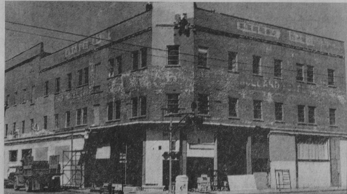
GETTING a fresh coat of paint is the old Holland Hotel at East Tawas, which is being remodeled and refurbished by a group of Saginaw investors. The front entrance of the famous hostelry is being remodeled and returned to the same location as when the building was originally constructed in the 1890s.
