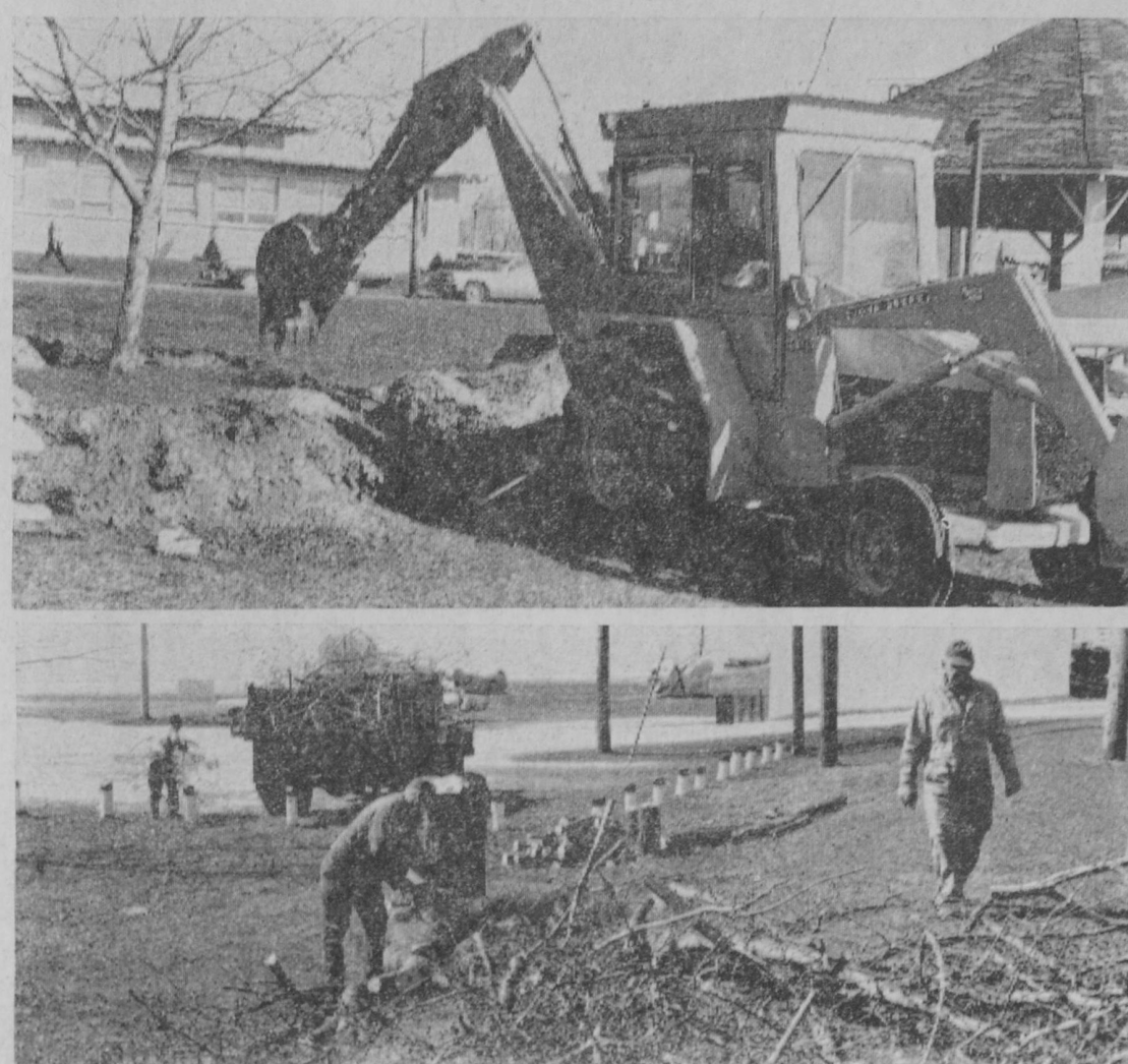
WORK STARTED MONDAY on preparing the Tawas City Park for expansion of the parking area along US-23. Three trees were moved to new locations by the Tawas City Department of Public Works and two trees, too large to handle,
