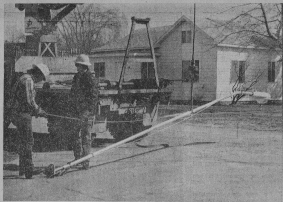
WORK started last week by Consumers Power Company on modernizing Tawas City's street lighting system. The program includes replacement of 23 2,500-lumen incandescent street lights with 6,500-lumen mercury vapor lights on First Avenue, from First Street to M-55; Fifth Avenue, from Mathews Street to M-55; Ninth Avenue, from the railroad tracks to Fourth Street; Oak Street, from the railroad
