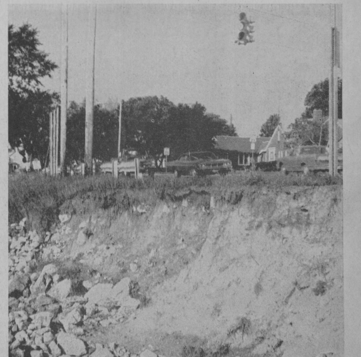
EROSION along Tawas Bay is endangering the roadway of US-23 near the M-55 intersection in Tawas City. Riprap protecting one area of the highway washed away about five weeks ago and City Mgr. Reginald Bublitz notified the Alpena office of the Michigan Department of State Highways. Danger to the roadway became even more
