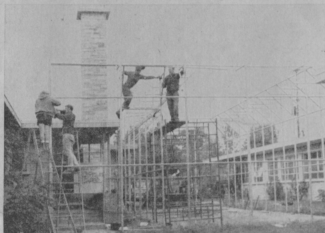
CONSTRUCTION on a new prisoner recreational "bullpen" at the Iosco County Jail is pictured here. Located at the former main entrance to the jail, the recreational area is situated in the court separating the jail and the county building. Construction of such a facility was a requirement imposed upon the county recently by the state jail inspector following an inspection of jail facilities here. Windows of offices of the county treasurer and register of deeds overlook the "bullpen" and a spokesman for the sheriff's department said that the facilities would only be
