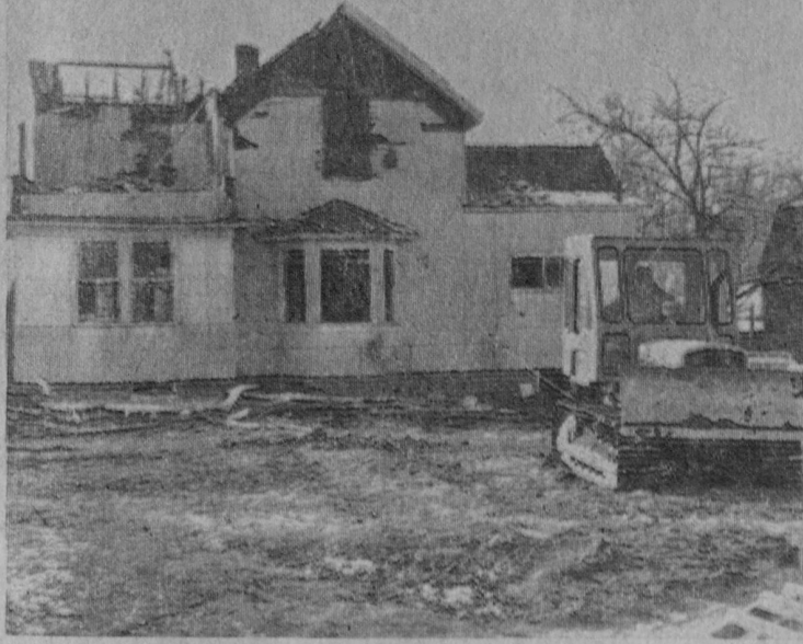
ANOTHER OLD HOUSE along US-23 (Lake Street) in Tawas City was demolished over the week-end to make room for commercial expansion. James Quarters is shown using his bulldozer to pull down the former residence of Robert Erickson, located near the North Street intersection. The house was once the dwelling of the late Mrs. Capitola McCormick. The site will become the new location for Tawas Hardware and, once the clearance is completed, work will start on the new building. It is expected that the new structure will be completed next spring.—Tawas Herald Photo.
