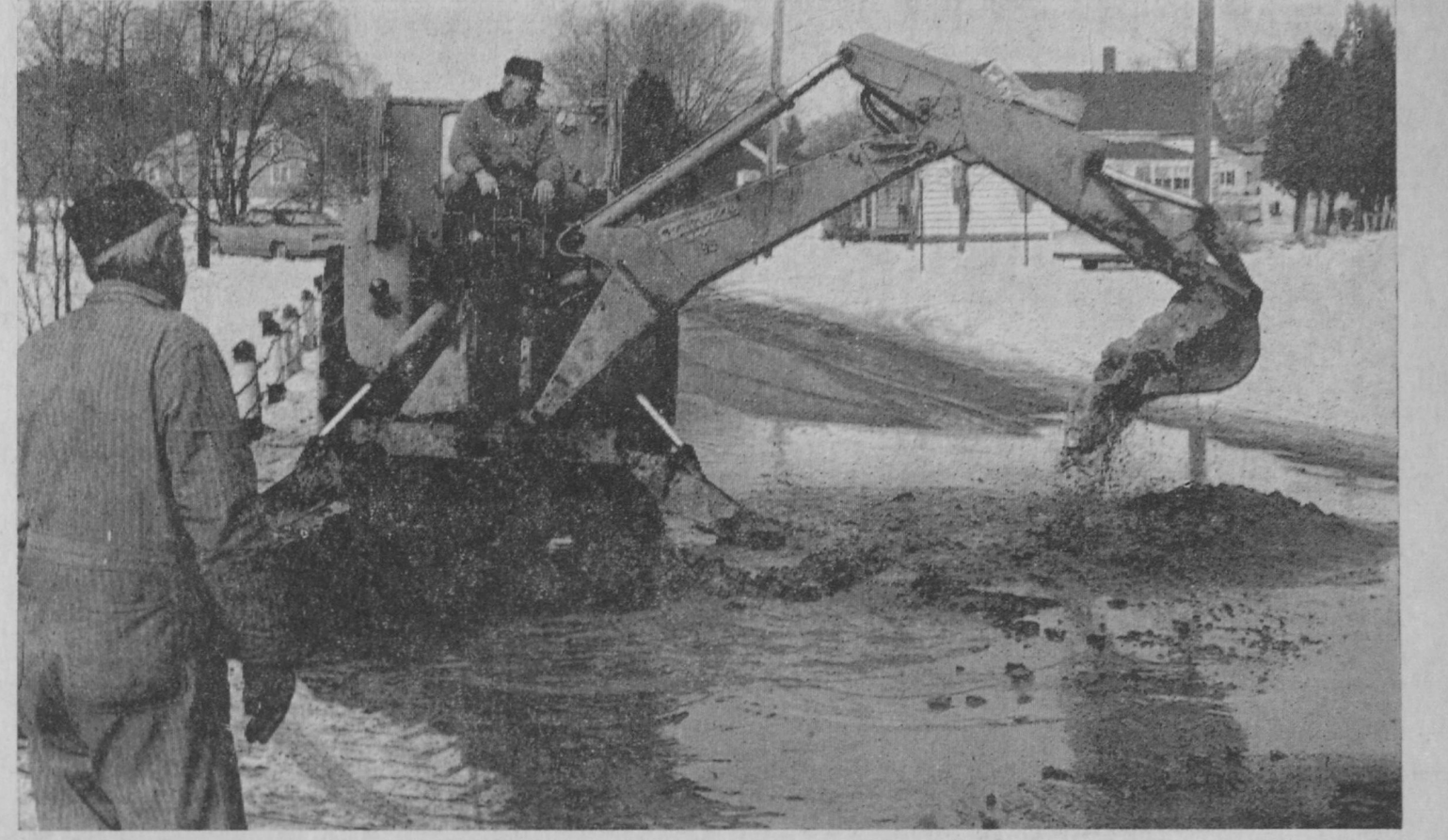
FROST PENETRATION caused a break in a water main Friday afternoon on Harris Avenue in Tawas City. Although water main ruptures are not uncommon in this part of Michigan during the winter, it was the second time in recent weeks that the Harris Avenue water main had to be shut down for repairs. As a result, water service to the Iosco Medical Care Facility and Tawas Area High School was disrupted while repairs were made to the water main by the Tawas City Department of Public Works. Afternoon
