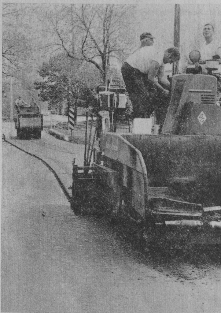
WITH A BREAK in the weather late last week, paving of Tawas City's major streets moved along rapidly. Equipment of Central Paving Company of West Branch is shown here on Sixth Avenue crossing the Dead Creek bridge. Rain early last week delayed the project. It is expected that the entire job will be completed this week.—Tawas Herald Photo.
