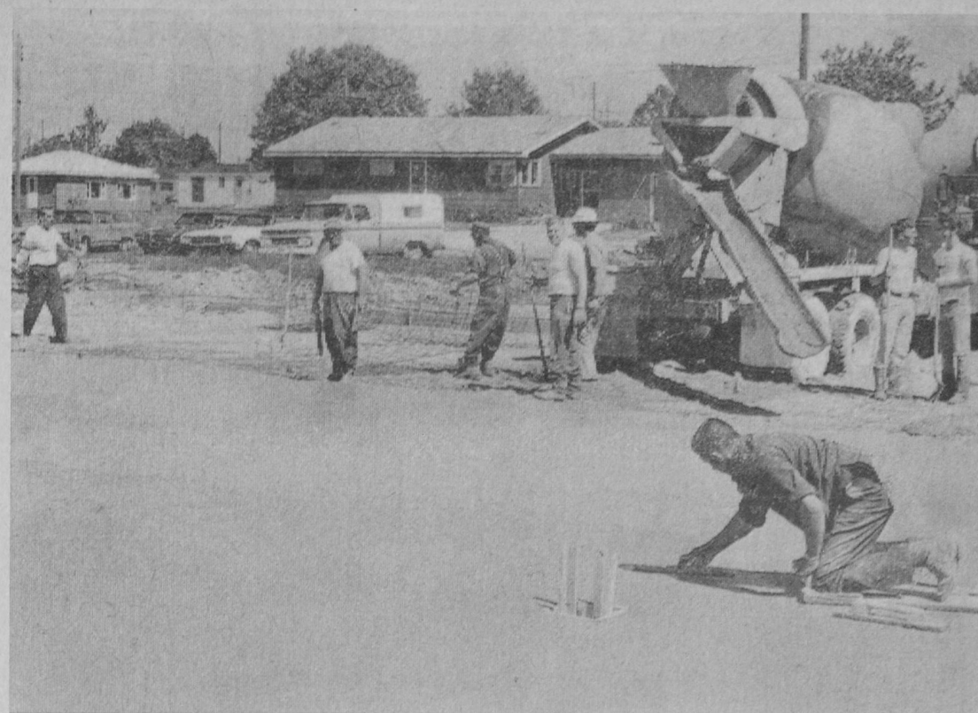
SIXTEEN VOLUNTEERS turned out Saturday morning to pour concrete for combination tennis-basketball courts and a winter ice skating rink at the new Whittemore recreational area on O'-Farrell Avenue. Construction of the 118 by 144-foot concrete slab is part of a $12,500 project undertaken by the Whittemore Fire Department
