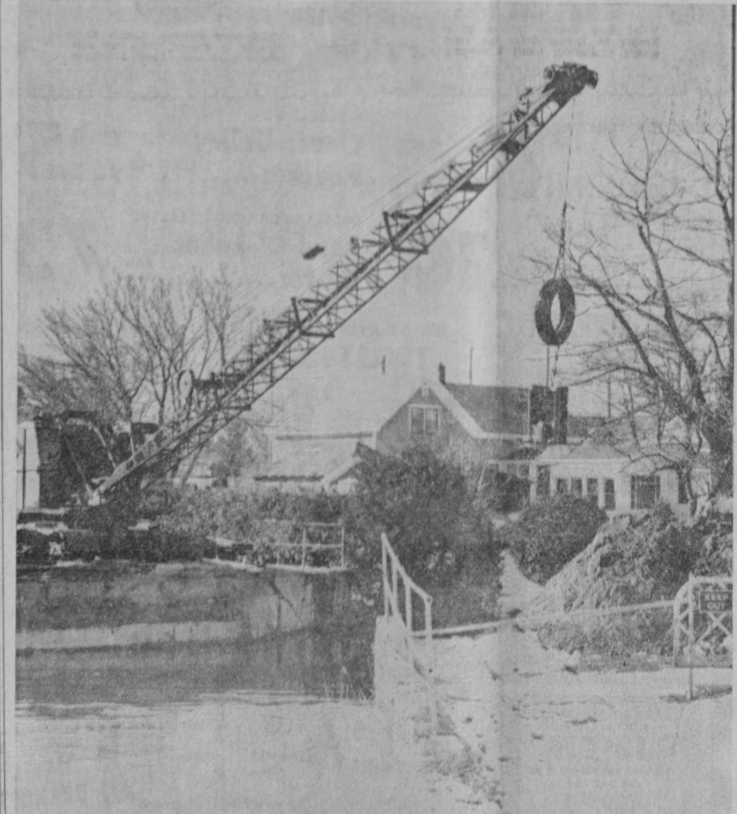
BY MONDAY AFTERNOON, the First Street bridge had been removed and the contractor for the City of Tawas City was busy using a dragline to remove a concrete retaining wall. Work is expected to start this week on driving piling into the river bottom for the new bridge.—Tawas Herald Photo.
