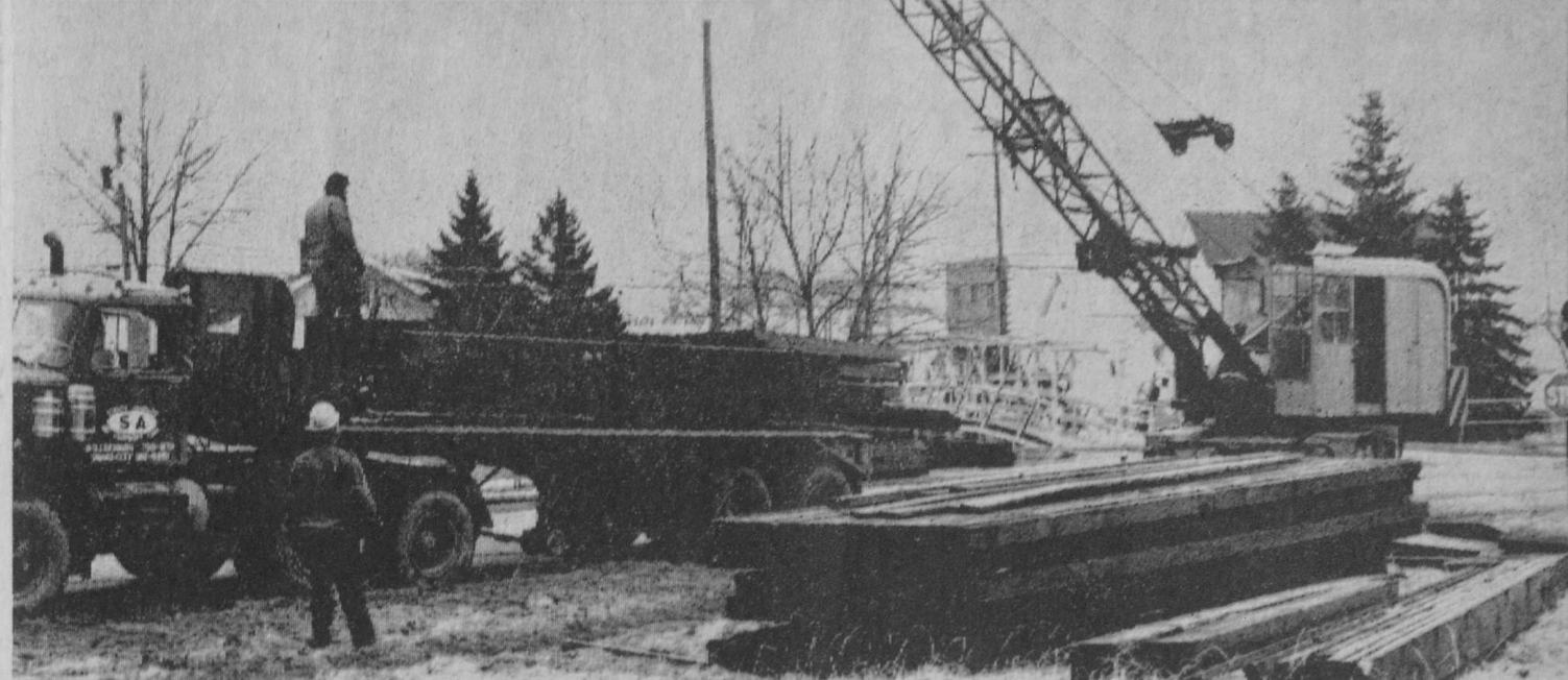
CONSTRUCTION is to start this week on Tawas City's two new wooden bridges at First Street and Mathews Street. Part of the material for the Mathews Street bridge is shown being unloaded above. A decision had not been reached Tuesday on which bridge would be constructed first as the city is negotiating for additional property on the south side of First Street. However, high water in the Tawas River may force the issue as one retaining wall on the old First Street bridge is eroding rapidly.—Tawas Herald Photo.
