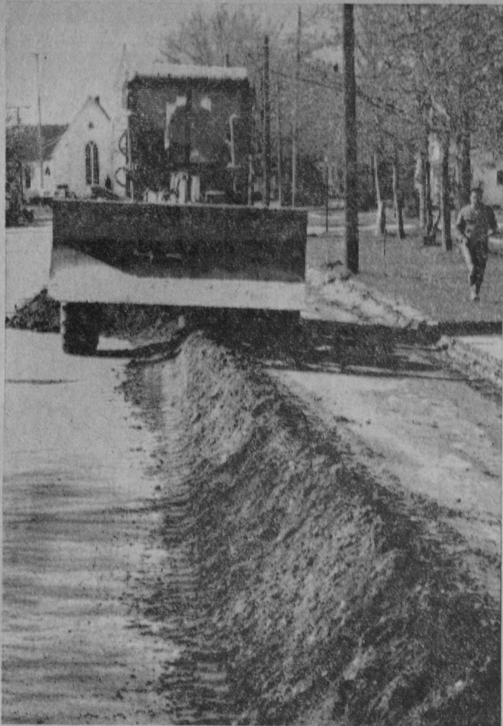
WORK started Monday morning by contractors for the City of Tawas City in grading shoulders along major streets of the city in preparation to receive a plant mix blacktop surface. The project, being financed through federal revenue sharing money, is to be completed in June.—Tawas Herald Photo.
