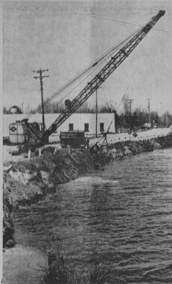
WITH COMPLETION of the new wooden bridge crossing the Tawas River at First Street, contractor for the City of Tawas City has moved to the mouth of the Tawas River where work has commenced on constructing a retaining wall along Ninth Avenue. High water in the bay, coupled with deterioration of the old retaining wall constructed in 1950, endangered Ninth Avenue with erosion of the west river bank. A new wall is to be constructed using treated timbers and piling. When this project is completed, the contractor is to move to Mathews Street to begin construction of a new wooden bridge at that point.—Tawas Herald Photo.
