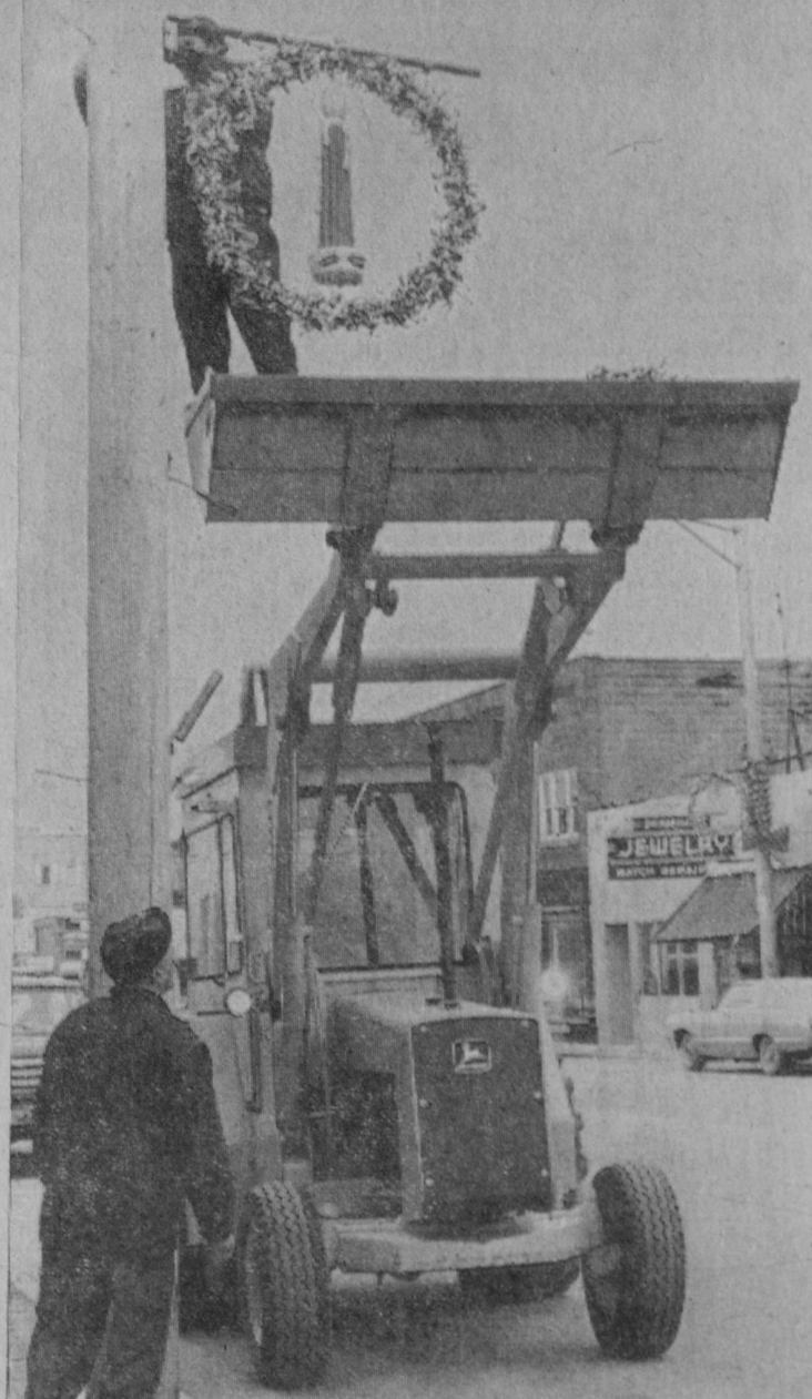
EMPLOYEES of the East Tawas Department of Public Works installed Christmas decorations on electrical poles along Newman Street Wednesday, but colored lights are to be used sparingly due to the energy crisis. A decision was to have been made at last night's meeting of the Tawas City Council regarding installation of Christmas decorations. City Mgr. Reginald Bublitz said Monday that street decorations and a lighted tree may be omitted this year due to the energy crisis.—Tawas Herald Photo.
