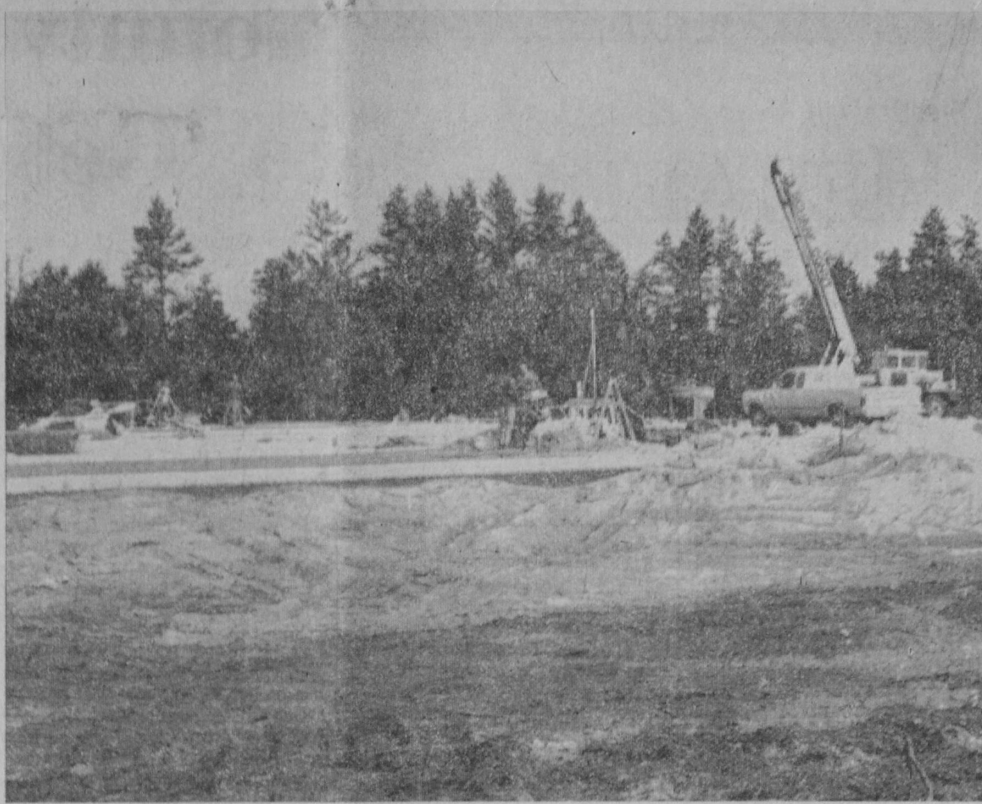
NOW UNDER CONSTRUCTION at the Tawas Area Industrial Development Corporation's park in Baldwin Township is this new building for Almo Manifold and Tool Company, which will manufacture hydraulic control manifolds and valves. Construction of this new plant will add new employment to the area, which has increased by 280 jobs since active promotion and development by the IDC.—Tawas Herald Photo.
