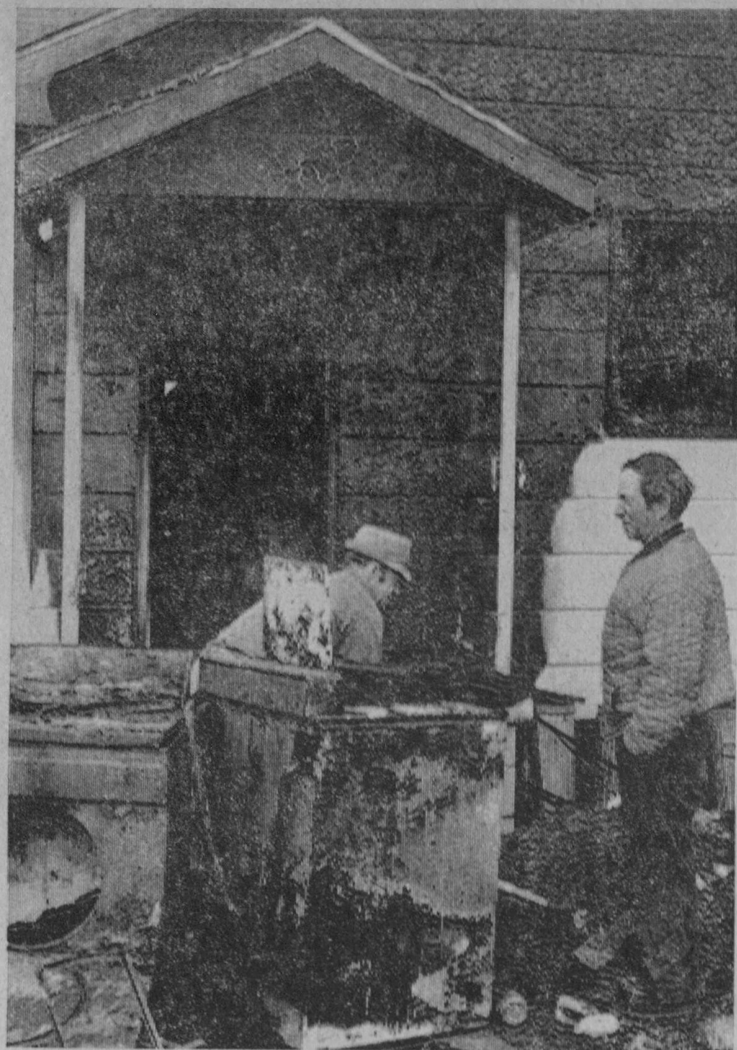
INSPECTING the damage to his home Monday morning following a fire is Charles L. Nash of 200 Adams Street, East Tawas. A washer and a clothes dryer removed from the utility room following the blaze are in the foreground. Intensity of the heat is evident from the charred siding and woodwork on the house. Clair A. Nash, brother of Charles, was assisting with the cleanup.—Tawas Herald Photo.
