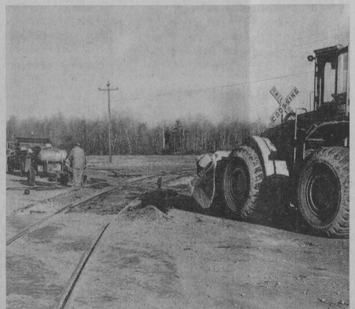
WORKMEN were busy Wednesday morning constructing a new crossing on Whittemore Road south of National City at the railroad spur line serving the National Gypsum Company quarry, Originally constructed about 15 years ago, the private railroad grade was below the level of the county road and was dangerous to vehicular traffic.—Tawas Herald Photo.
