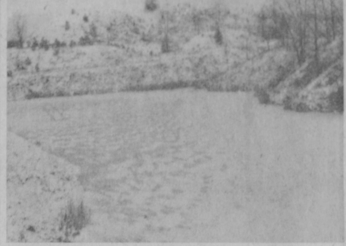
AN IMPORTANT part of the operation is to beautify the area which has been mined. One area is to be terraced for a future housing development and a number of lakes are being created.
