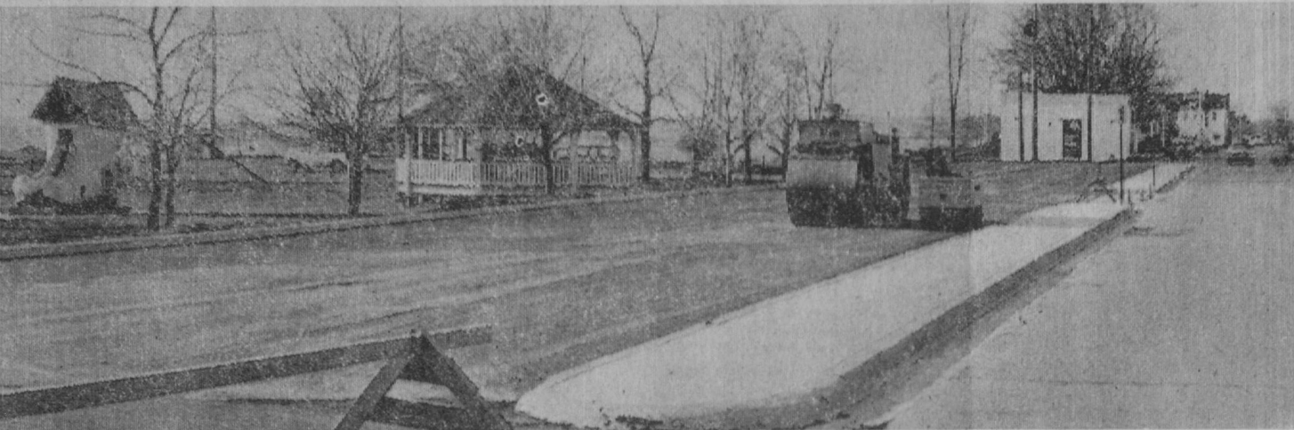
THE CITY OF TAWAS CITY completed a major street blacktopping and bridge construction program during the year, along with expansion and hard surfacing of parking facilities at the city park.
