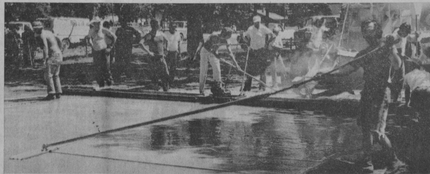
VOLUNTEERS of Grant Township pitched in Saturday to construct three new concrete tennis courts near the fire hall at Sand Lake. This is part of a recreational facility being planned under sponsorship of the Grant Township Fire Department. Aiding with financing the tennis courts was a grant from federal revenue sharing money received by Iosco County. All of the labor was donated.
