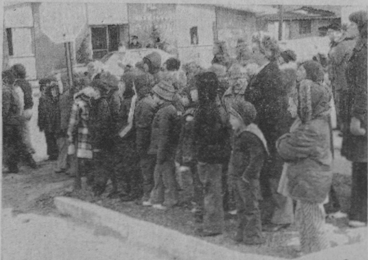
TRAFFIC STOPPED, people gawked and cameras clicked Monday morning as workmen set a new steeple in place on Christ Episcopal Church, East Tawas, which is now undergoing reconstruction. A large boom truck was used to hoist the steeple roof more than 50 feet into the air and set it in place. Spectators included school children (bottom photo) who were dismissed from class to view the operation. The top photo looks through a small opening in the top of the steeple roof, which was lifted off the ground by means of the steel rings in the foreground. The steeple was being inched into place in the center photo. The church is to observe its centennial this summer.—Tawas Herald Photos.
