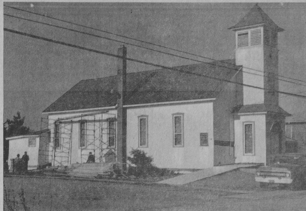
WORK ON REMODELING St. James Catholic Church at Whittemore is expected to be completed in early June, according to the Rev. Fr. Terrence Raymond, pastor. Interior of the church has received new pews, carpeting and a new furnace. The building has been lowered two blocks in order to facilitate construction of a covered concrete ramp entryway. Workmen are
