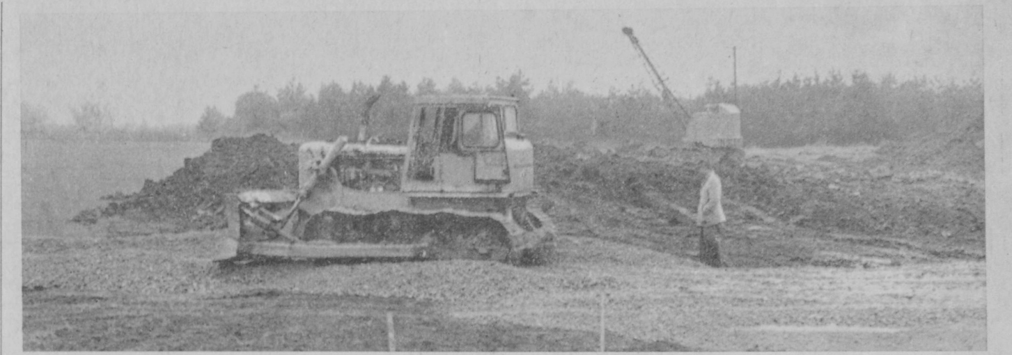
COUNTY ROAD COMMISSION equipment is shown here working on a new entrance road to the site of the proposed new county garage east of Sand Lake Road and south of M-55. The site is to be used as a temporary gravel stockpile area.—Tawas Herald Photo.
