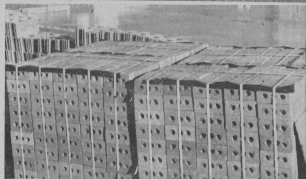
PROGRESS on the new Hale Baptist Church is shown in these photos. Construction is running ahead of schedule, according to a spokesman for Hale Home Center, contractor, and the new church is to be ready for occupancy by Christmas. The top
