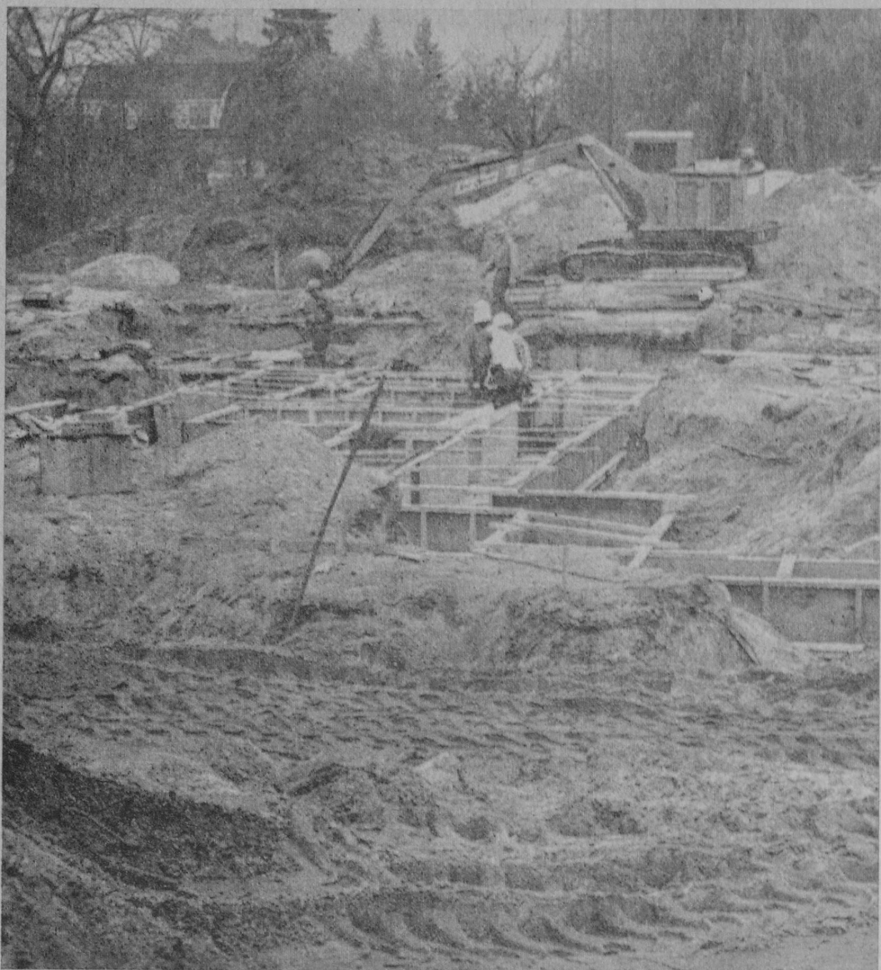
PROGRESS on construction of footings by Gregory Construction Company, Bay City, general contractor, for the new federal housing apartment building at East Tawas is shown here. The picture was snapped Tuesday morning and shows workmen preparing forms to receive concrete. The building is to provide 41 units of low rent housing for the elderly and is located at the intersection of Church Street and Bay Street.—Tawas Herald Photo.
