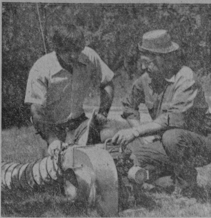
PREPARING to use this smoke machine on one of Tawas City's sewer mains are Barry Burke, left, Edmonds Engineering Company, and Buryl Binder of the city's department of public works. Smoke was forced into the mains to determine points of infiltration of storm water.—Tawas Herald Photo.
