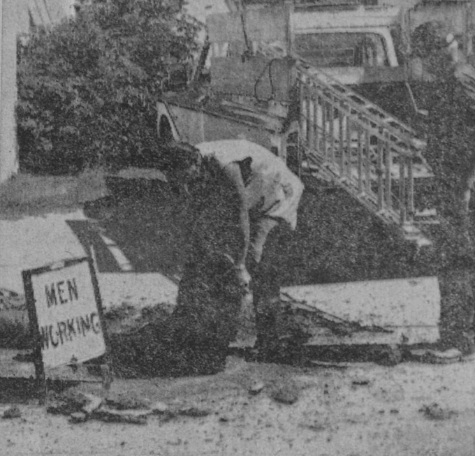
MEMBERS of the department of public works crew are shown above opening a manhole on First Street in preparation to test a sewer main.—Tawas Herald Photo.
