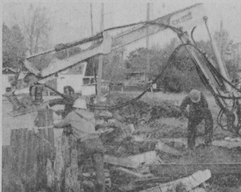
Steel sheeting was installed on the pier at the Tawas City Park.
