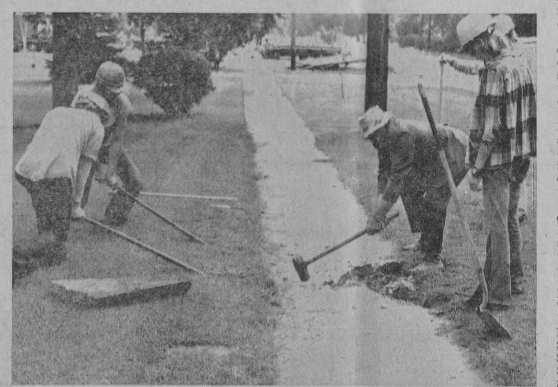
SWINGING a sledgehammer in the above photo is Vernon Eckstein, veteran Tawas City contractor, who has been hired by the City of Tawas City to act as advisor on a federal-locally sponsored sidewalk construction program. The federal CETA program provides funds for hiring unemployed students to work on the project and one member of the city crew, Bruce Fisher, is assisting.—Tawas Herald Photo.
