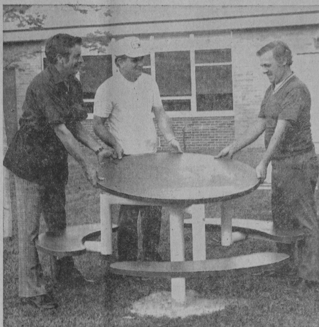
INSTALLATION was completed Wednesday evening by East Tawas Lions Club on six new picnic tables at the Tawas City Elementary Unit. According to Herman Rollin, principal, the tables are to be used for outdoor classroom purposes. The all steel tables cost $1,800. Shown working on the project from left are Joseph Sergent, Charles Palmer and Joseph Chaisson. A plaque installed on the south wall overlooking the courtyard is shown in the lower photo.—Tawas Herald Photos.
