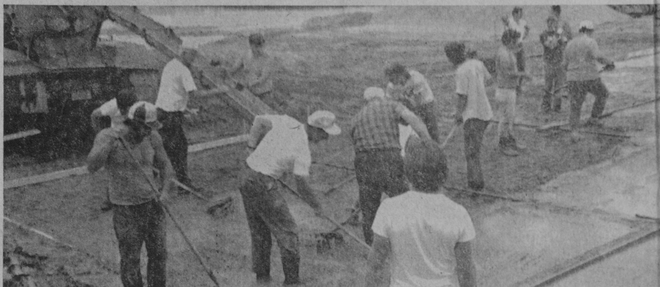
At least 25 Hale area volunteers were on hand all day Tuesday, June 24, to work in wet concrete.—William Wereley Photos.
