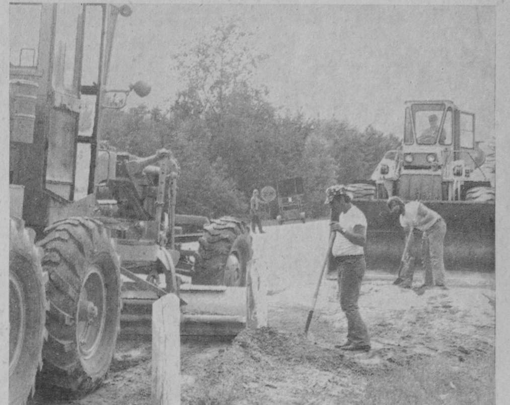
WORK STARTED THURSDAY on grading work along the north shoulder of M-55 from the US-23 intersection west to Plank Road for a bicycle route. The project, announced earlier this year by the Michigan Department of State Highways, is
