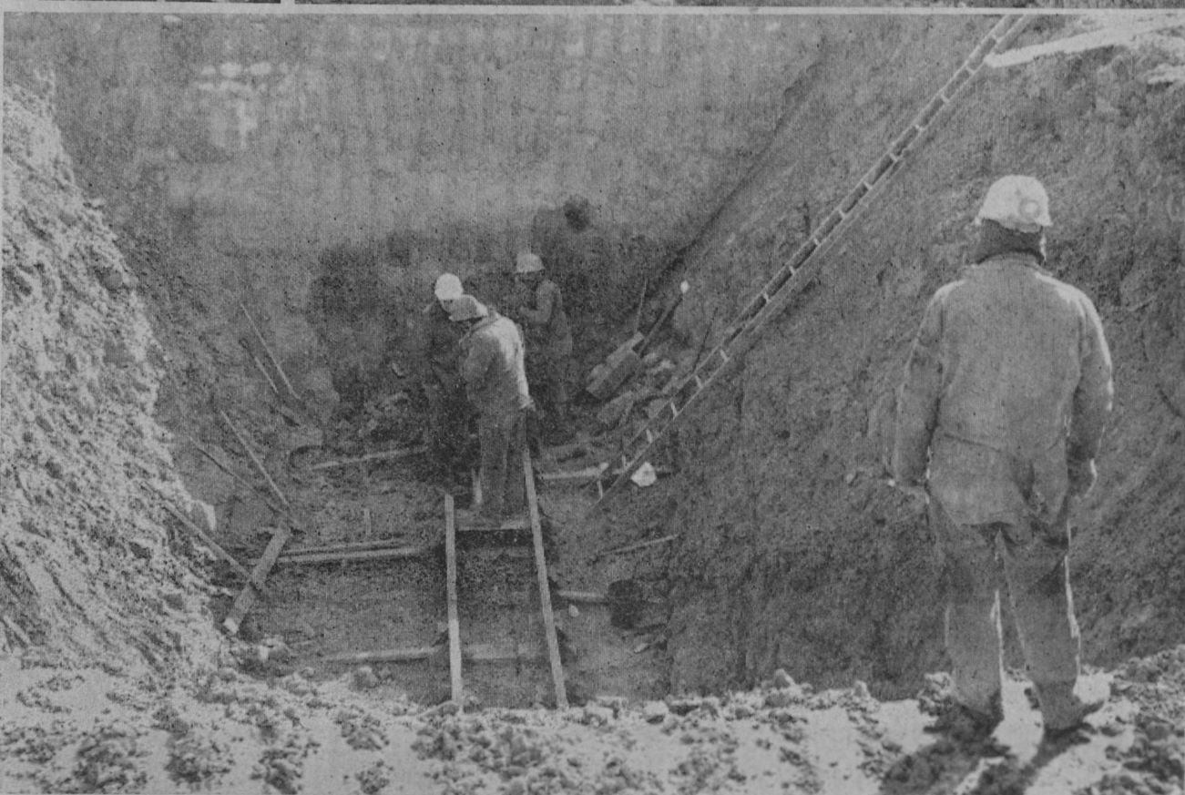
WORK STARTED last week on construction of a little more than two miles of sanitary sewers in Tawas City. This project, much debated and often controversial in preliminary stages during the past 1½ years, will provide sanitary sewer service to the last major areas of Tawas City presently lacking sewers. T. A. Forsberg of Okemos, low bidder on the project, started excavation work for installation of mains along US-23 (shown in the photo at top right) and made a deep excavation east of First Avenue (lower picture) and began boring
