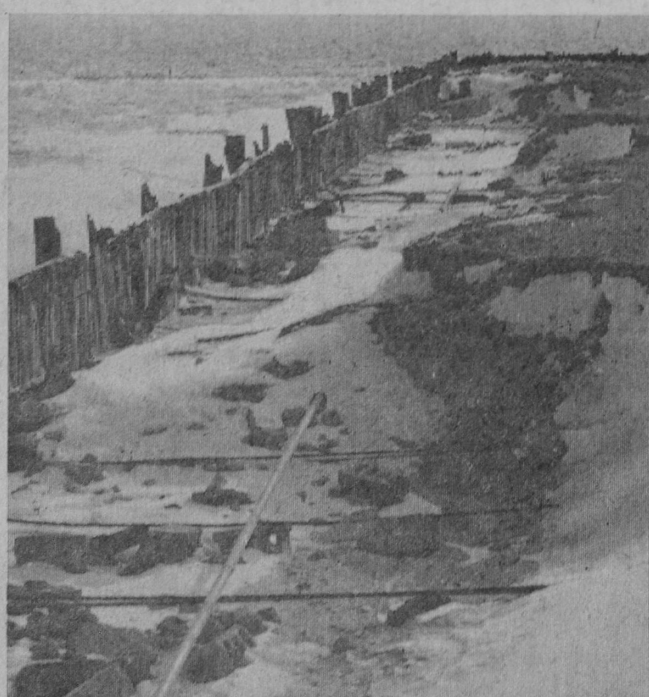
THE PIER in the Tawas City Park looked like this last year when the City of Tawas City received a permit from the Michigan Department of Natural Resources to make repairs using sheet steel. Work has been completed on the first phase of the project, but the city has been cited by the United States Army Corps of Engineers for failing to get a federal permit before work began.—Tawas Herald Photo.
