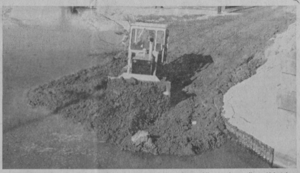
A BULLDOZER was at work Monday afternoon pushing clay into the Tawas River in the first step toward repair of a water main break under the river. Freezing weather is necessary to hold the clay in place while workmen dig a 13-foot-deep trench to locate and repair the ruptured main.—Tawas Herald Photo.
