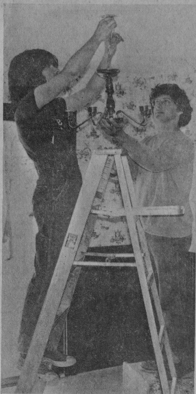
WORK on Tawas Area School's building trades house is nearing completion and the new dwelling will soon be offered for sale by the school. An open house is to be held Saturday and Sunday, May 31-June 1, in order to show work of the class. Gary Steed, left, and Bernard Link, right, are shown installing a light fixture. Turn to page 6, section 2, for more pictures.—Tawas Herald Photo.
