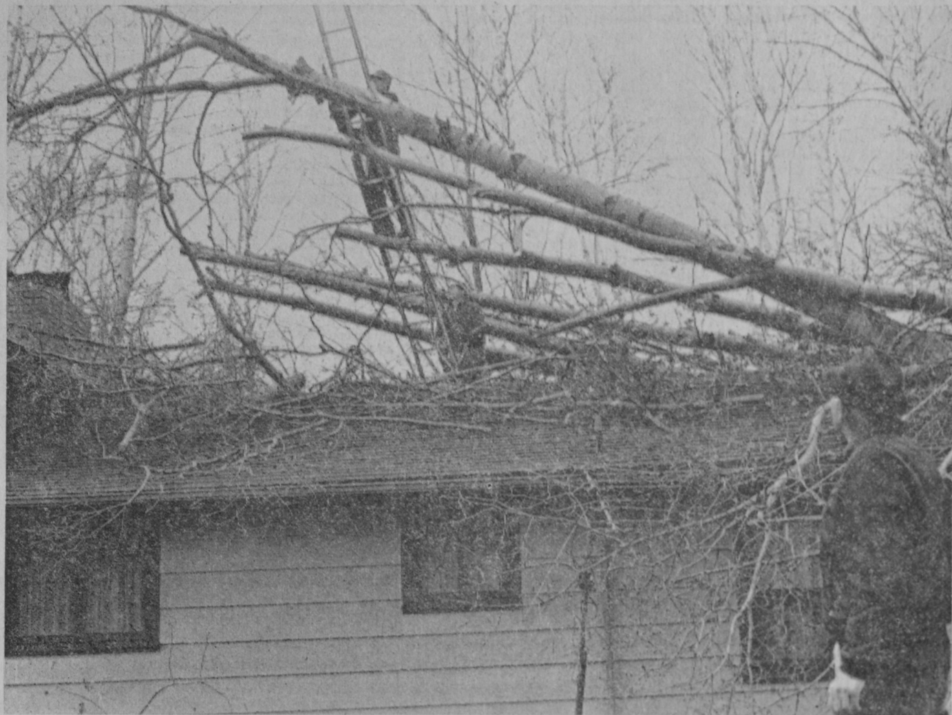
IOSCO COUNTY was fortunate to escape last week's tornado with minimal damage as compared to an estimated $500,000 to $750,000 damage just over the west county line in Ogemaw County. Six confirmed touchdowns by twisters were reported in the Long Lake area near Hale. Several homes were damaged by twisters or fall-
