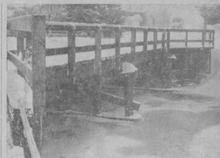
A WOODEN BRIDGE over the Tawas River at Mathews Street is near the site of the first lumber mill on the Lake Huron shore between Bay City and Mackinaw.—Tawas Herald Photo.
