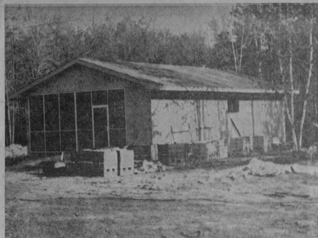
PROGRESS on the new post office building at National City is pictured above. The new building is located about one mile east of Jordan's Store, present location of the post office. George Jordan said the move into the new quarters is expected around July 1. The building is being constructed by Custom Home Builders of Houghton Lake, building owner, and is to be leased to the postal service. The 24 by 42-foot structure is to have a brick exterior.—Tawas Herald Photo.
