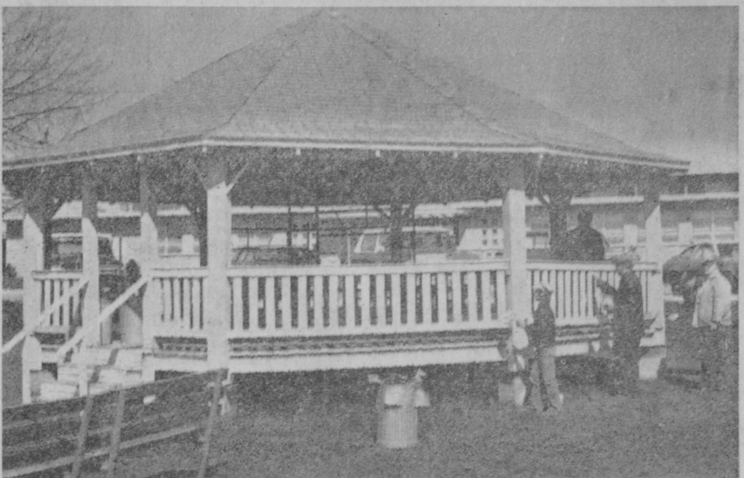
TAWAS KIWANIS CLUB has completed its project of restoring the band stand in the Tawas City Park. Members of the club volunteered to paint the old structure and building trades students of Tawas Area High School installed a new roof, replaced roof and floor boards and repaired railings. Materials were donated by area
