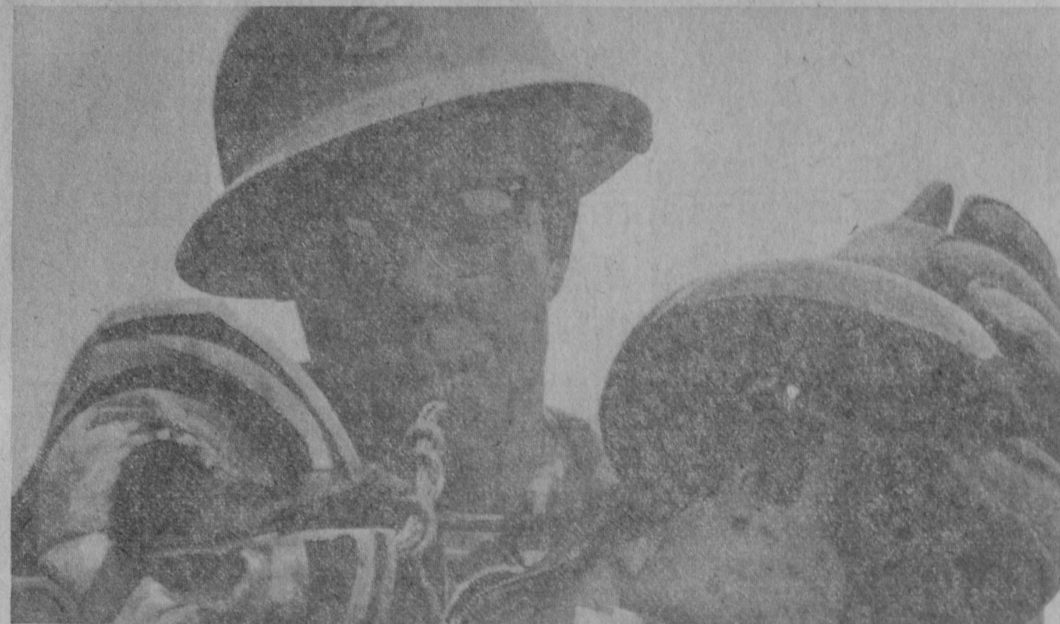
DAMAGE CONTINUES —An insulator from an 11,000-volt Consumers Power line is inspected by John W. Knight, a company electrical serviceman, after a gunshot damaged it and caused 272 customers to be without power for six hours. Repairmen had to walk the line to find the damaged insulator. The company offers a substantial reward for information leading to the arrest and arraignment of, or restitution from, any person damaging insulators. It cost the company's customers $100,000 to replace insulators damaged by gunshots last year.
