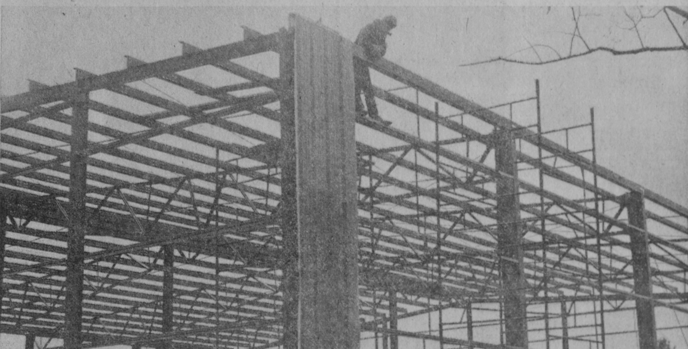
BOPP-BUSCH Manufacturing Company currently is constructing a new steel warehouse building across Industrial Avenue from its tool and die division in Tawas City. Workmen were in the process
