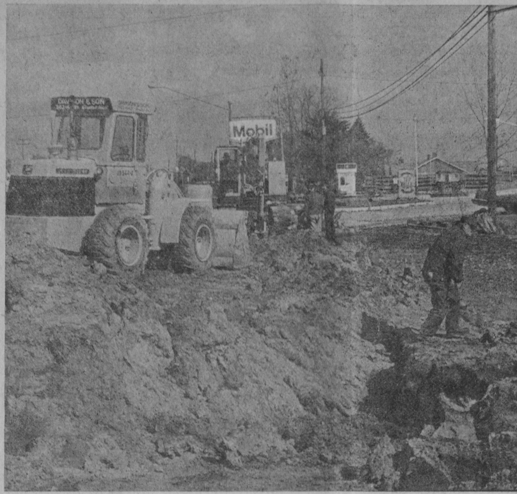
WORK STARTED last week on constructing the special assessment sanitary sewer along US-23 from the Tawas River bridge south to Acapulco Beach Cabins. Authorized by the city council after public hearings and acceptance of a special assessment tax roll, the city was notified two
