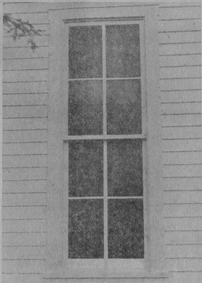
ORIGINAL IDEA of the bicentennial committee was to replace narrow windows shown above. It was found that siding and the roof had deteriorated and the project was expanded.—Tawas Herald Photo.
