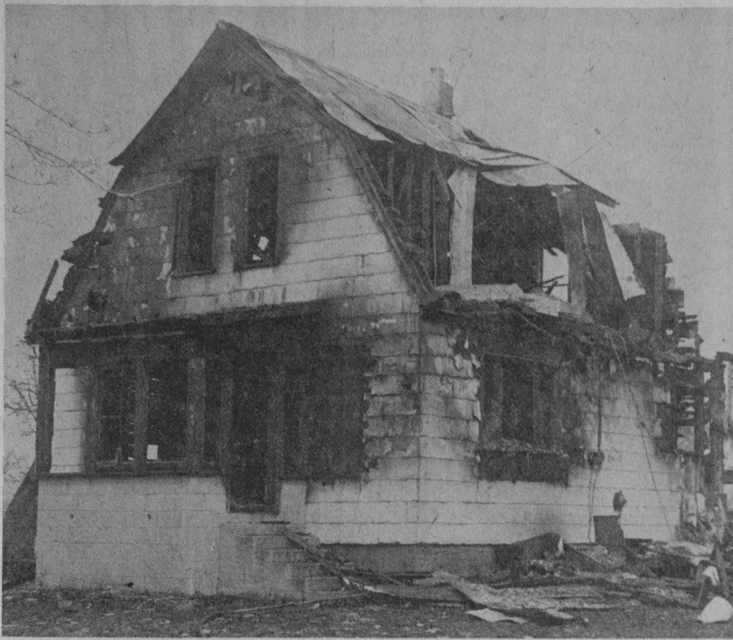
FIRE APRIL 12 left a family of five homeless in Plainfield Township. Mr. and Mrs. Larry Miller and their three children of Curtis Road, 2 1/4 miles west of Hale, lost everything when the blaze gutted this two-story house, formerly the John Harris farm. The blaze broke out about 4:00 p. m. and Miller used a garden hose in an effort to control the flames. Smoke filled the house and he could not see the numbers on the dial telephone and he could not recall the number of the Plainfield Township Fire Department. Miller
