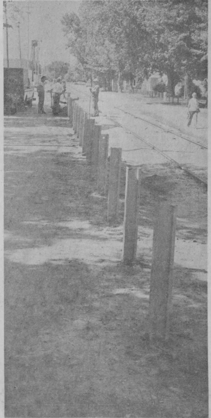
WORK started Monday morning on construction of a steel rail fence along Court Street. The above picture shows progress as of Monday noon.—Tawas Herald Photo.
