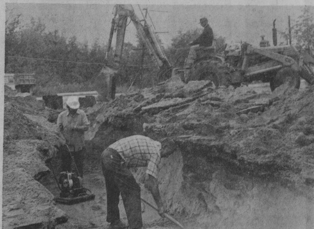
TRAFFIC on M-55 was detoured Monday in Tawas City following a cave-in during boring under the highway for construction of the area's water expansion project. The bore was completed Friday but seepage of ground water caused a washout. As a result, the contractor had to cut through the blacktop road surface and fill the trench.—Tawas Herald Photo.
