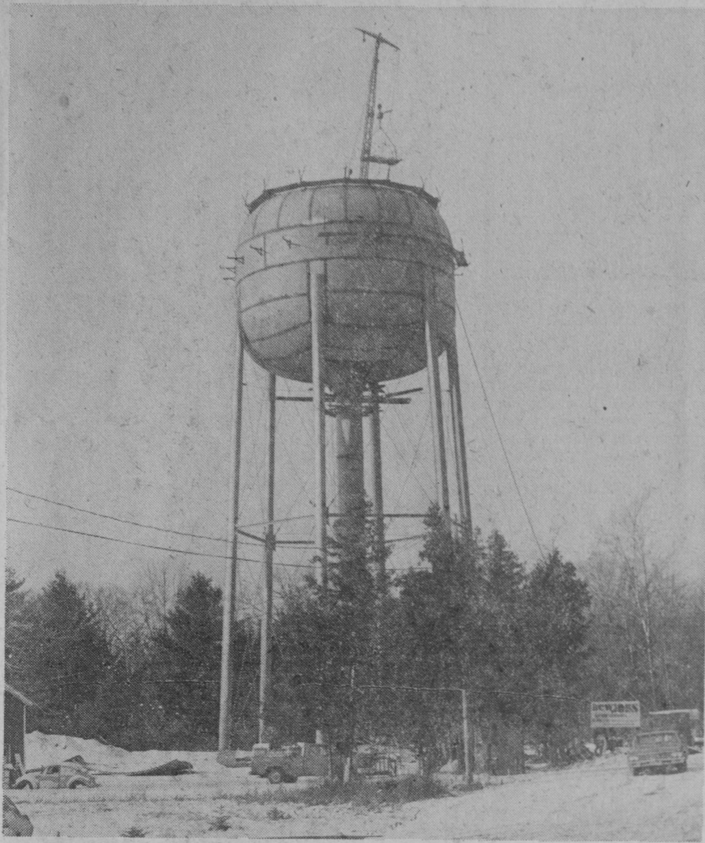
CONSTRUCTION on the 500,000-gallon water tank at the Tawas City industrial park is nearing completion. Although the tank will not be painted until next spring, Pittsburgh-Des Moines Steel Company is putting the finishing touches on welding the bowl. This tank, along with one at the industrial park on Aulerich Road, will provide pressure at each end of the Tawas area water system.—Tawas Herald Photo.
