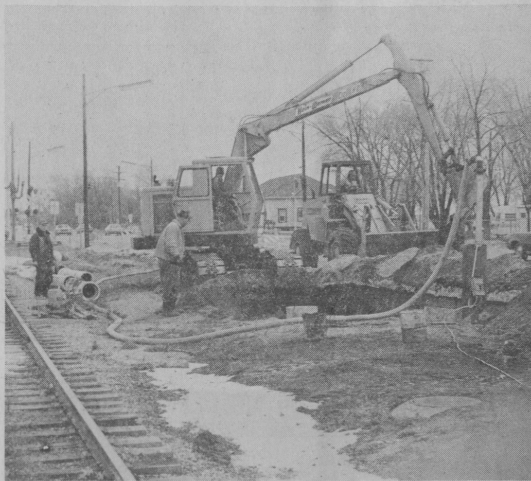
WORK CONTINUED last week on construction of a water main at East Tawas. Pressure testing and sanitizing is required before mains will be ready for use. Turn to page 6, sec. 2, for story.—Tawas Herald Photo.
