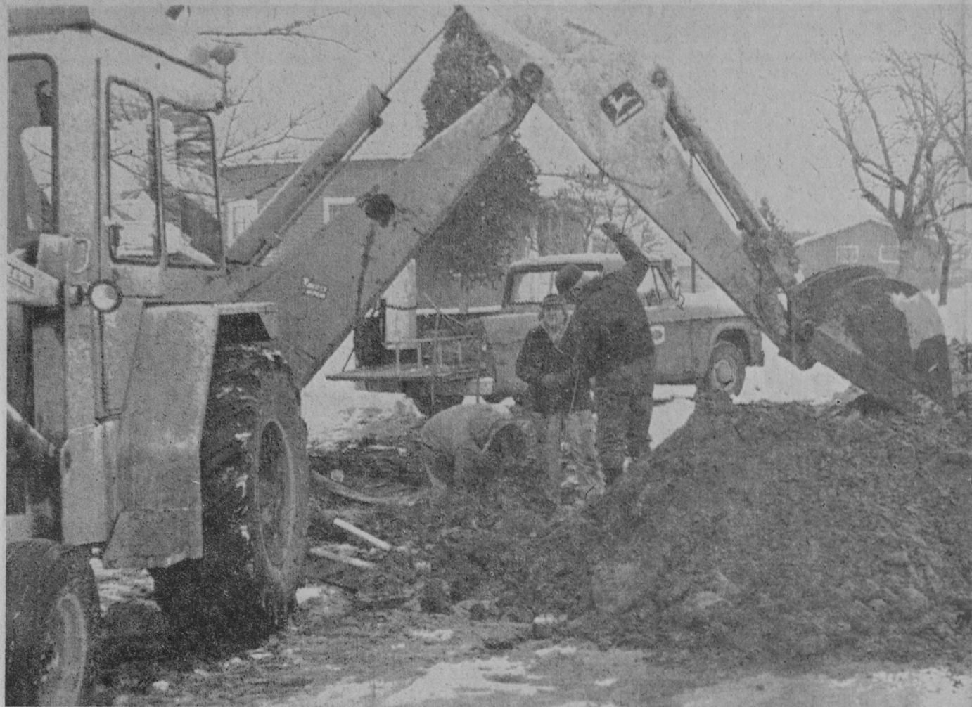
TAWAS CITY Department of Public Works spent six hours Monday repairing a water line break on Sixth Avenue. A second water line break occurred Tuesday on Ninth Avenue. A total of 12 water
