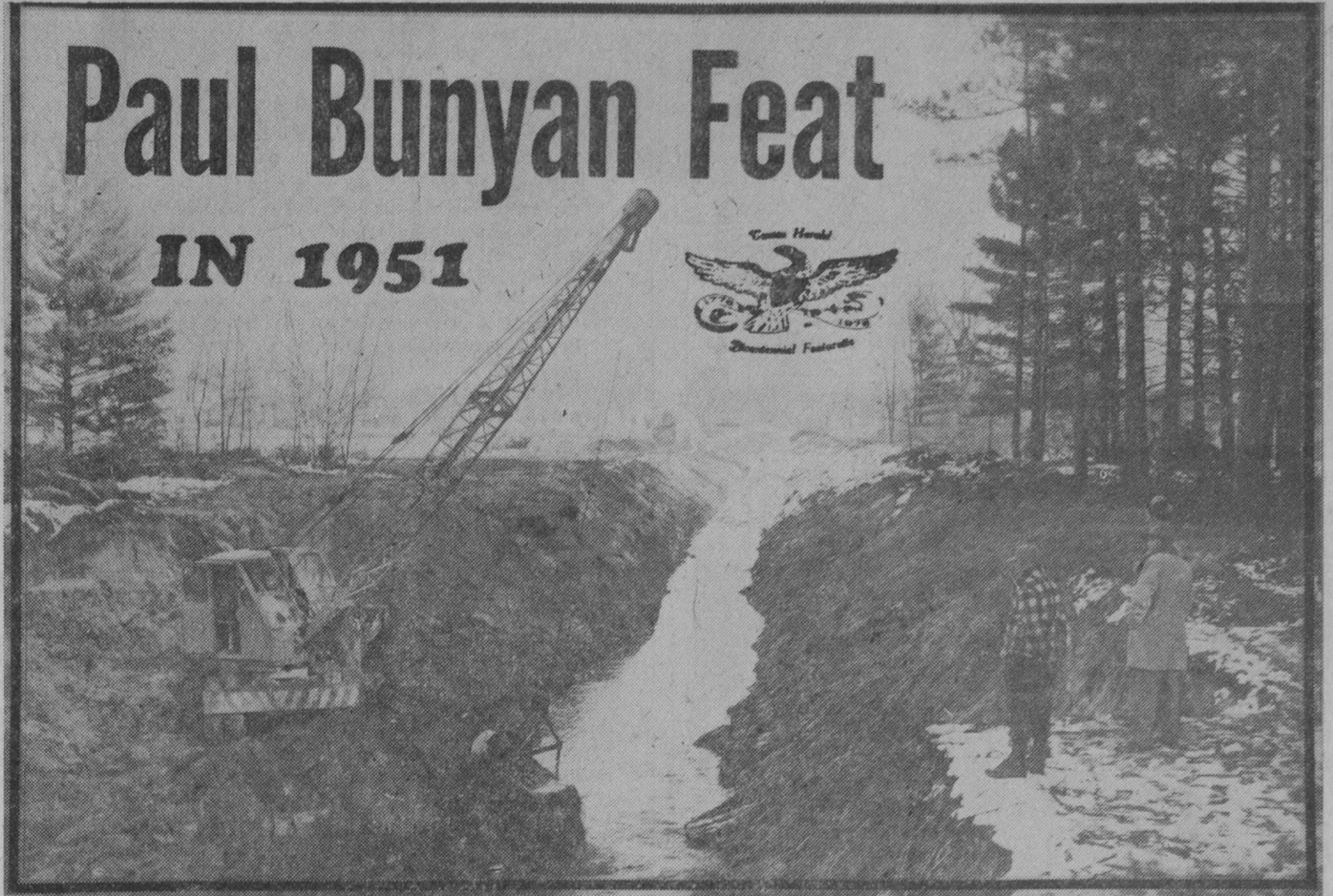
HISTORIC MOMENT on December 1, 1951, is recorded above when a dragline scooped the last shovelful of earth to open the new channel straightening the course of Dead Creek. Few residents
