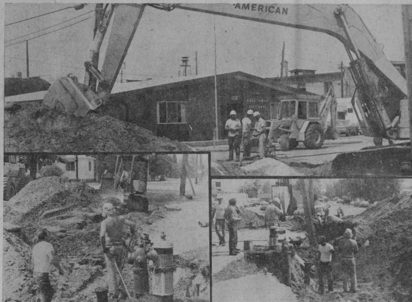
PROGRESS on construction of expanded water services in the Tawas and Baldwin Township is pictured above. Workmen of GGL Contractors, Belleville, are shown constructing a force main
