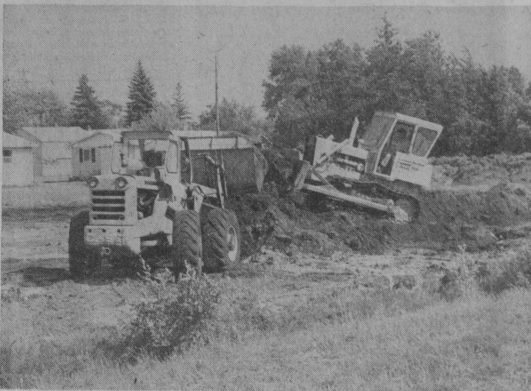
GROUND was broken last Wednesday by equipment owned by John Henry of East Tawas for the new Manitou Village apartment complex in Tawas City. One unit is expected to be completed by mid-November and a second is to be completed a month later.—Tawas Herald Photo.
