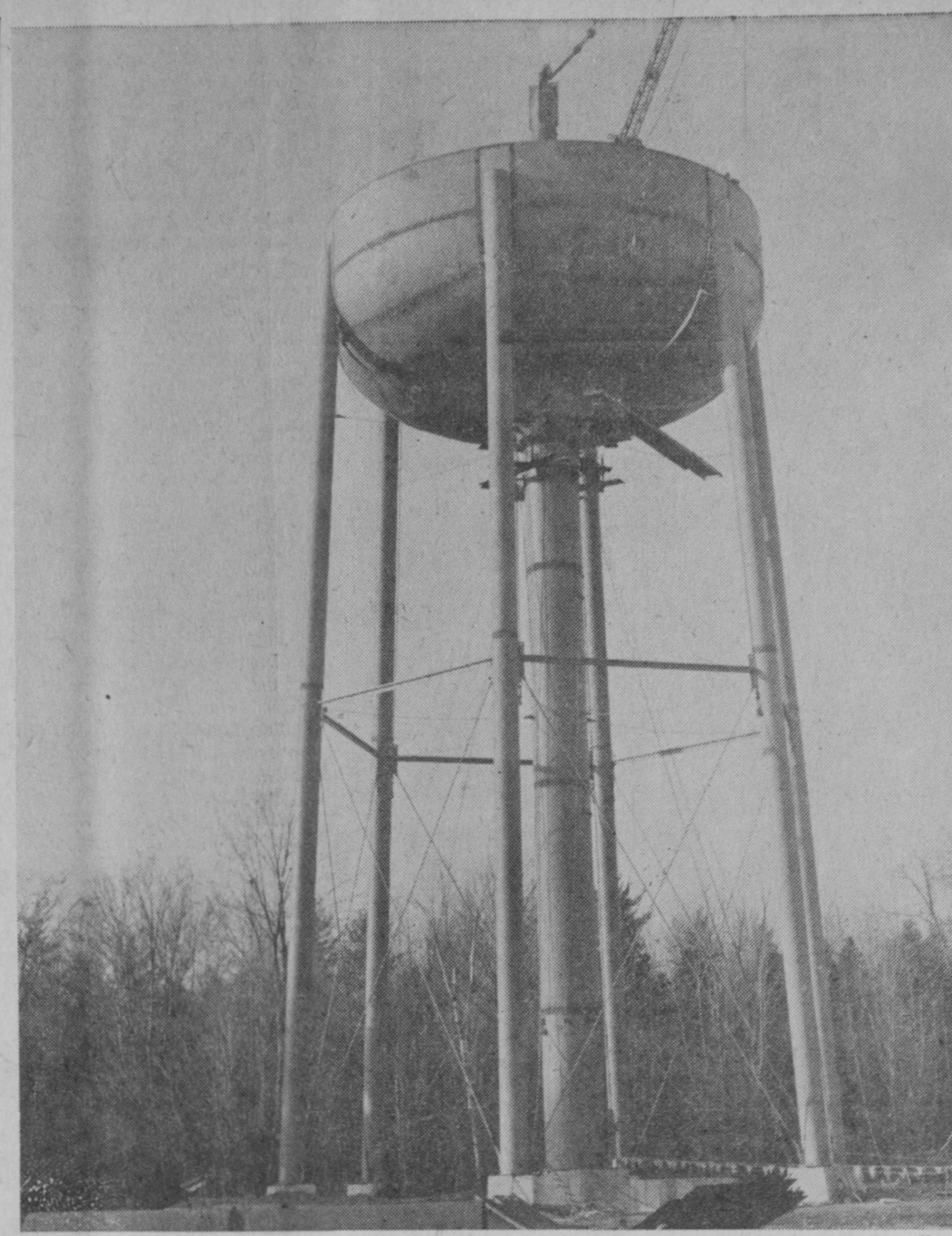
PROGRESS on construction of the new water stand pipe at the Ninth Avenue industrial park in Tawas City is pictured above. Workmen of the Pittsburgh-DesMoines Steel Company are currently welding the bowl of the 500,000-gallon water storage facility. A similar tank is being constructed at the industrial park in Baldwin Township.—Tawas Herald Photo.
