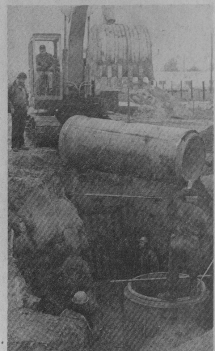
CREW of the Tawas City Department of Public Works was working in a trench about 17 feet deep Tuesday afternoon when this picture was snapped. A 32-inch concrete main is being lowered into place on North Street where a storm sewer has been under construction for the past month.—Tawas Herald Photo.
