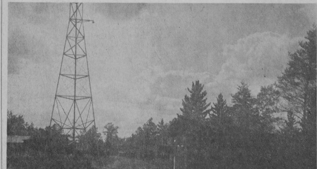
CONSTRUCTION of high tension power lines through Iosco County to reach the Saginaw Valley was opposed by numerous residents and Sherman Township rejected the power company's
